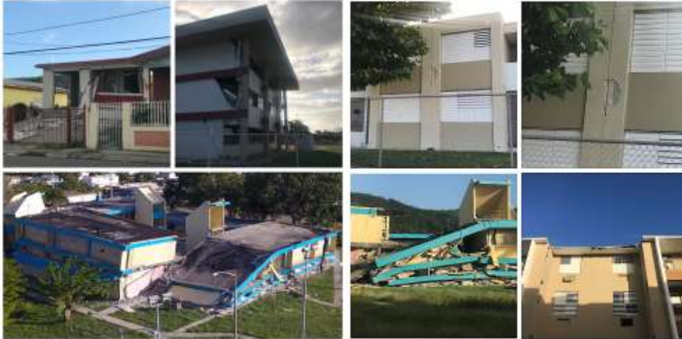
Image 4: Structures damaged in downtown Guánica (from left to right, house damaged, Departamento de la Familia, Residencial Jardines de Guánica, Escuela Intermedia Agripina Seda, Residencial Luis Muñoz Rivera.
